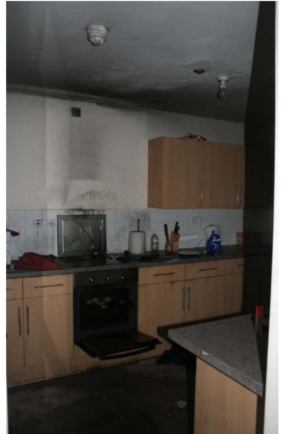
Above: The fire damage caused by a cigarette was localised and significantly reduced with the operation of fire
